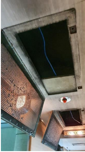
7. Swab Sample Location – Car 2374 Return Air Duct
